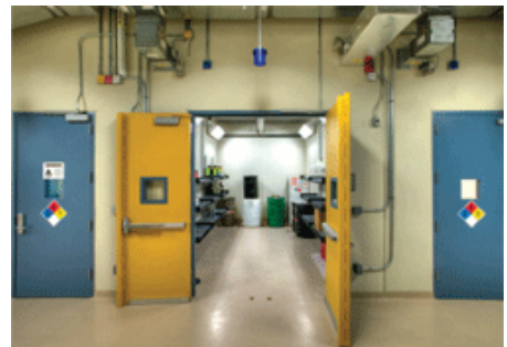
This view of a deflagration room shows that one door opens 90 degrees while the other opens 180 degrees. The interior face of the doors is painted bright safety yellow. This serves as a flag - when the room is in use, workers in the center of the facility will know where their buddy is, or that a room is not secured. Outside the room are a light switch and outlet devices, allowing control of the room from the outside.
