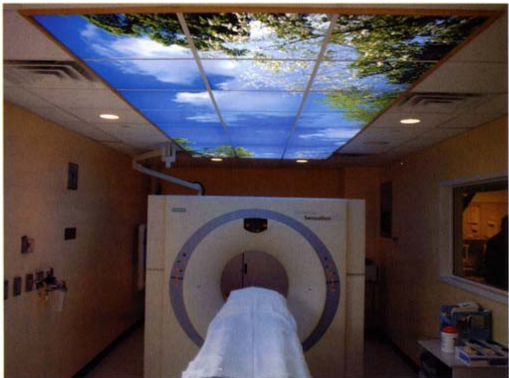
Sky ceilings offer designers an affordable means by which to bring the illusion of natural light into a windowless space.
